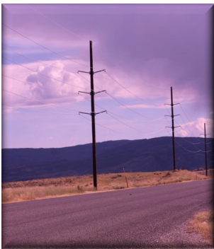
Heber Light & Power double circuit mono-pole sub-transmission line.
